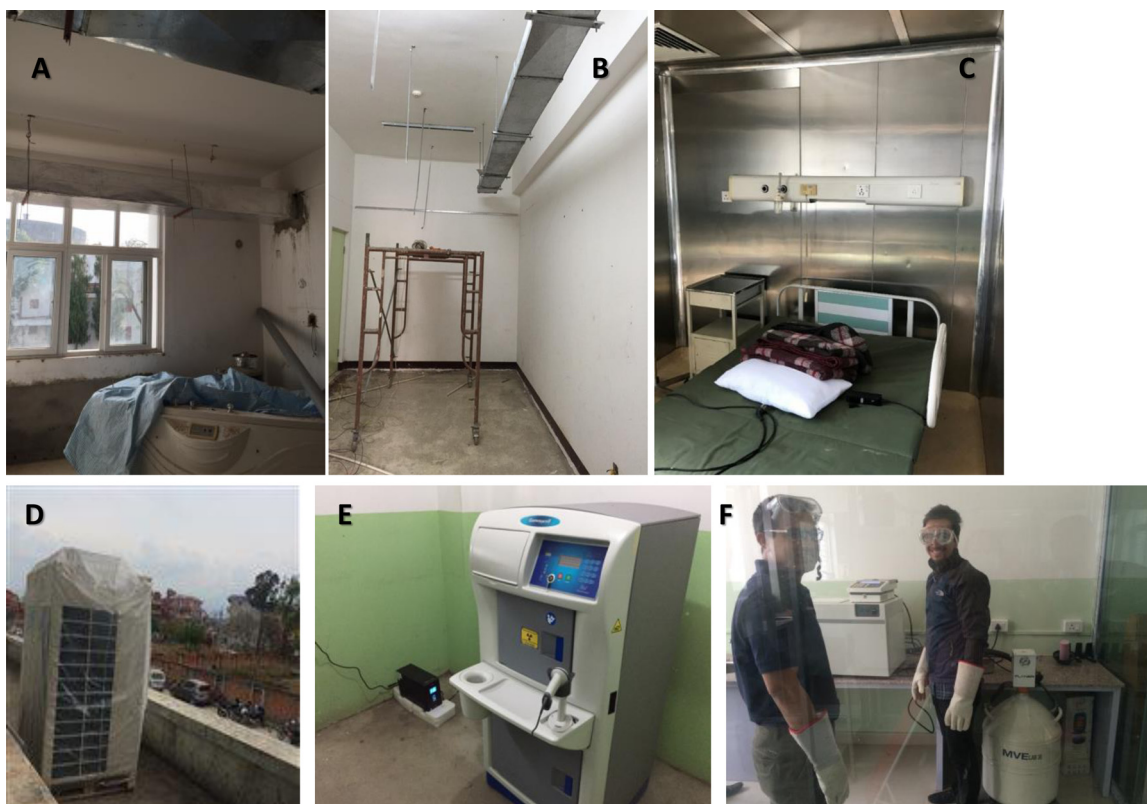
Figure 2. Building the BMT unit in phase 2 of the project. Intervention of local engineers during the construction of the BMT unit addressed the high risk of mold infection from the external walls of the old hospital (A) by reinforcing the wall structure (B) and applying metal internal panels in the patient rooms (C) and positioning the HEPA filter on the roof of the hospital above the BMT unit (D). During phase 2 of the project, the lack of irradiated blood products in Nepal was addressed by purchasing a dedicated irradiator (E) that was positioned inside the BMT unit. The same space included a separate cell processing laboratory with liquid nitrogen automated stem cell cryopreservation system (F), as well as a -80^{\circ}\text{C} freezer (not shown).
